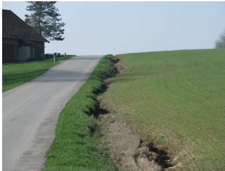
Erosion rill found during the field survey
