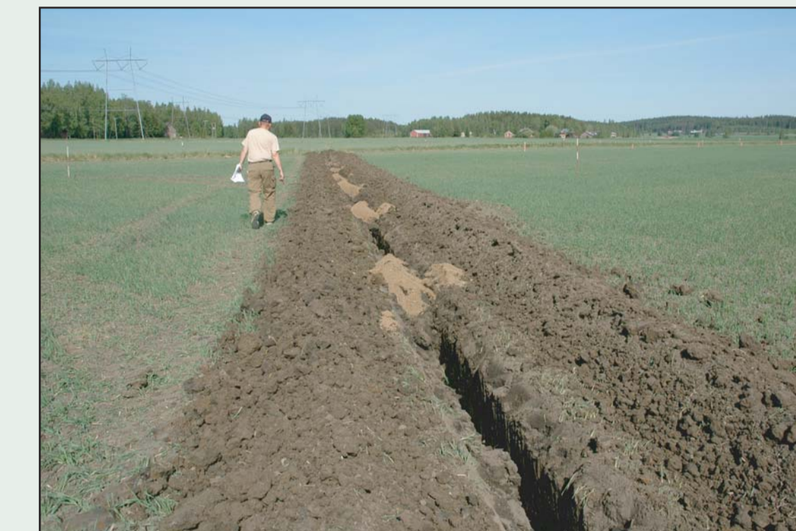
Gravel was filled to the top (blind inlet) every 8 meters. The trenched soil was left to dry for a week after which it was used to fill up the trench.
