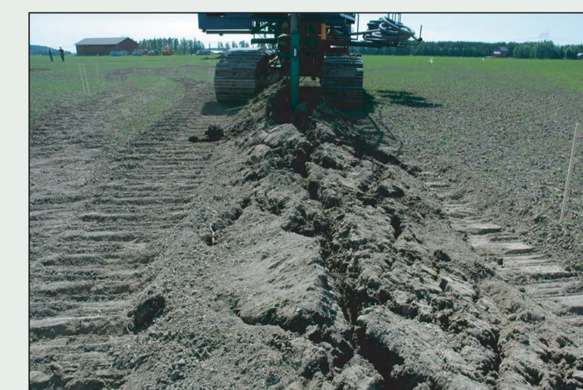
Drainage plow was used in this method. The trench closes right after the pipe laying.
