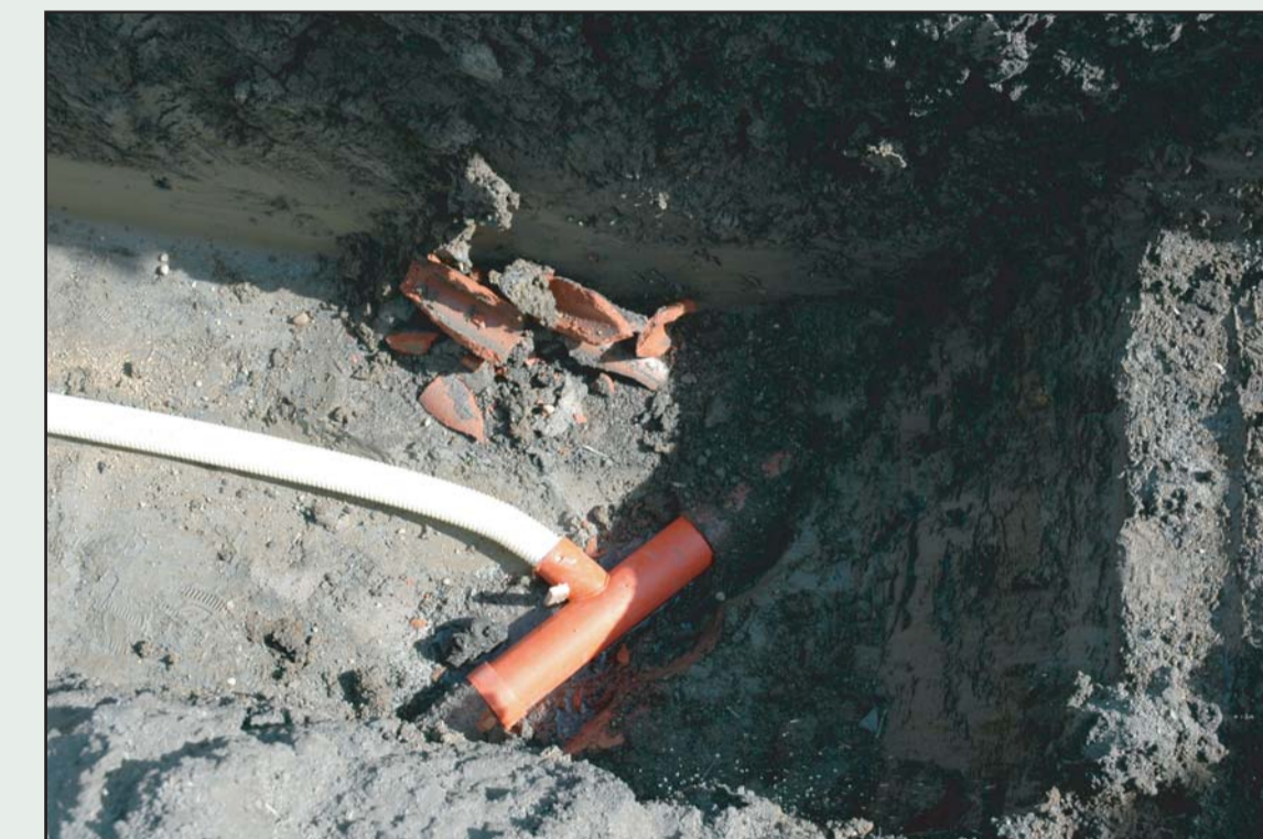
The new pipes were laid between the old ones and connected to the existing collector.
