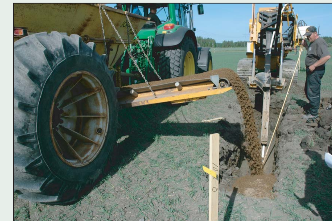
In method I the additional drainage was done with a drainage trencher, plastic pipe and gravel was used as envelope material.
