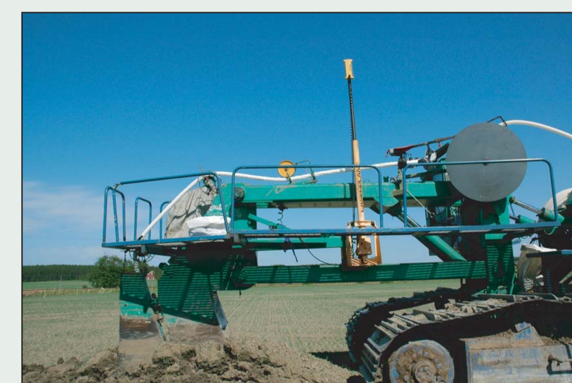
The drainage plow is equipped with a device that installs the envelope around the pipe on site before laying the pipe.
