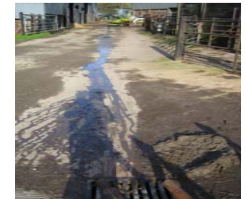
Fig 8. Contamination of clean water drain with dirty water
